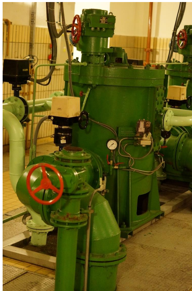
Hydroelectric power station Orlik
