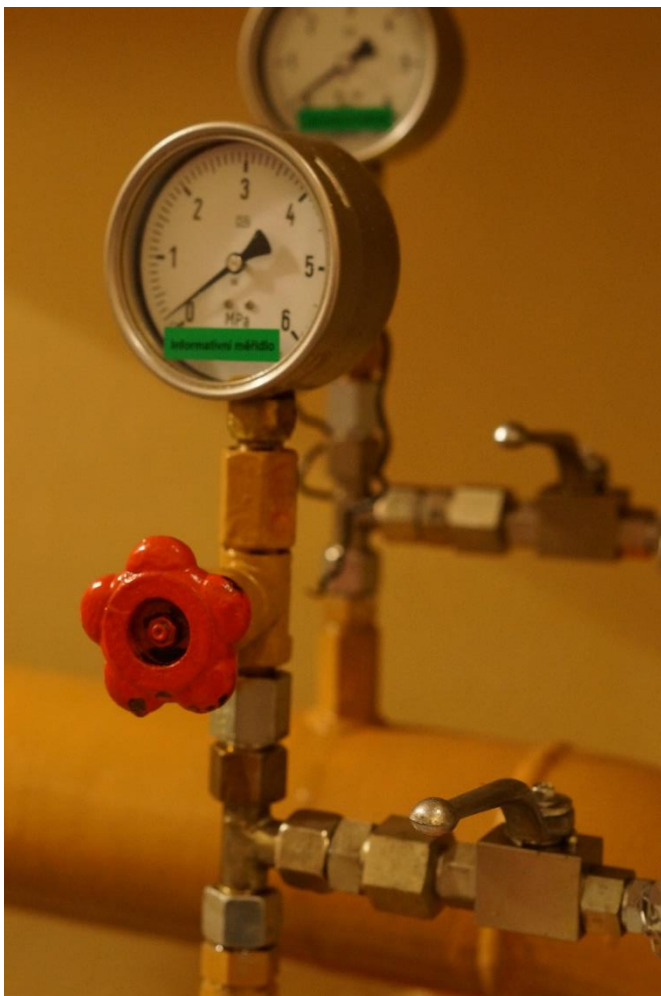
Hydroelectric power station Orlik
