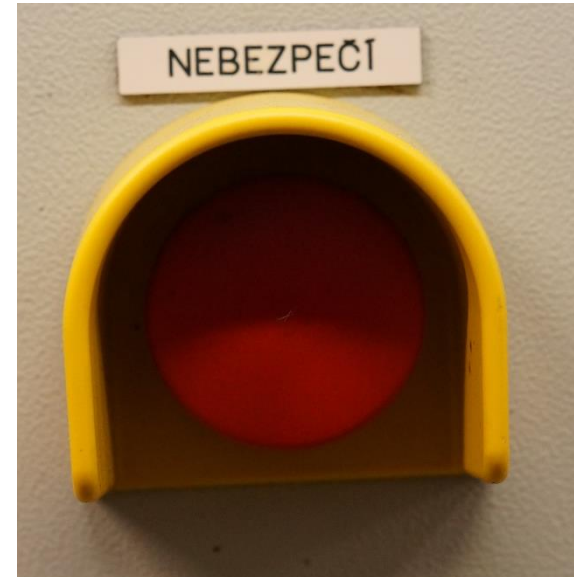
Hydroelectric power station Orlik
